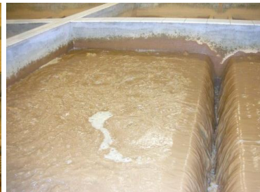
Sandfilter under skyl
